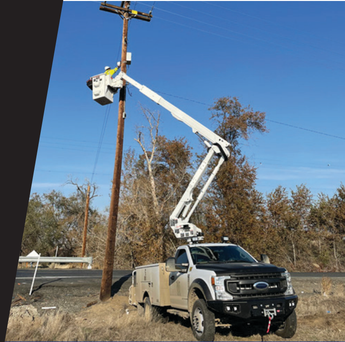
Installation of the MUST device along a rural road in Washington State. Source: Yakama Nation.
